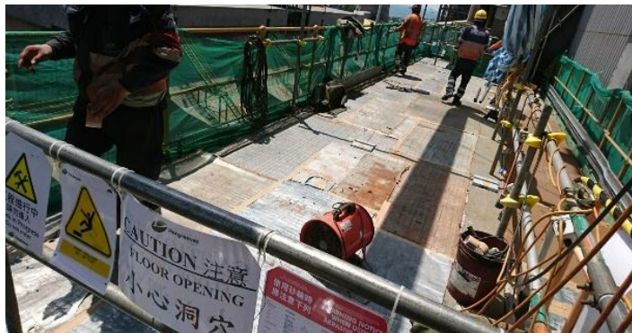
Proper barricade and display signage 適當圍封及展示警告標誌
